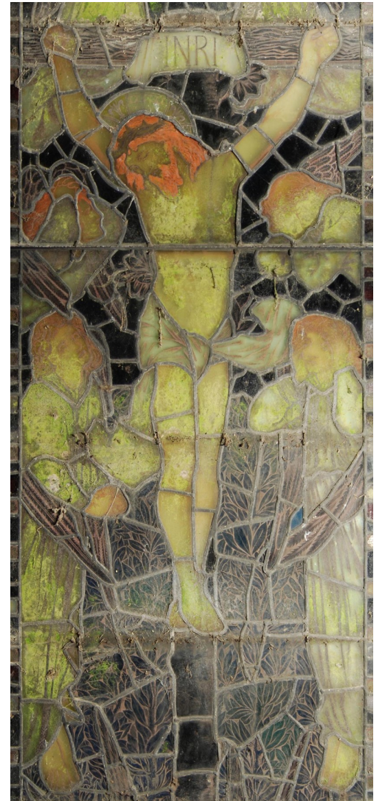
Green algae growing on glass surface due to damp conditions
