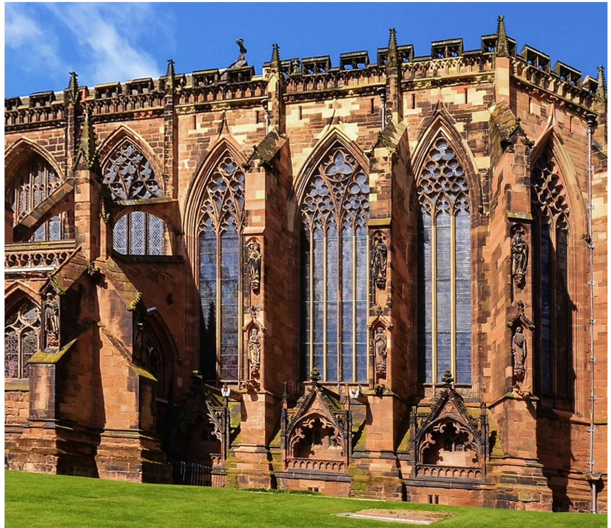
Lichfield Cathedral Lady Chapel, with Environmental Protective Glazing (full-pane, kiln-distorted glass) and wire guards protecting the world-famous 'Herkenrode' windows
